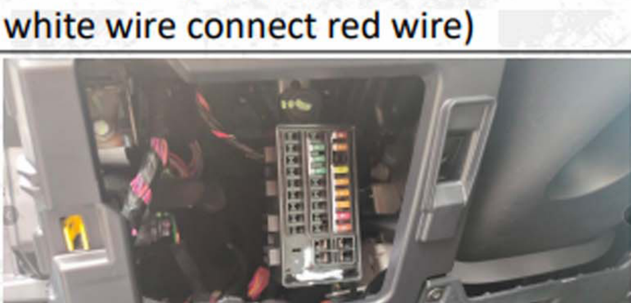
11. Find the main electricity in the safe box
